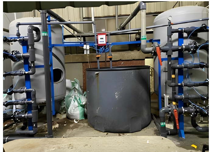
Duplex Water Softener with Multivalve System
