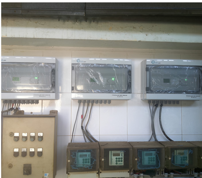
East Antara Water Treatment Station Geziret El Dahab Water Treatment Station
