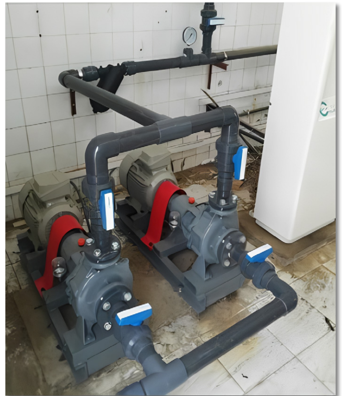
Badrasheen Water Treatment Station
