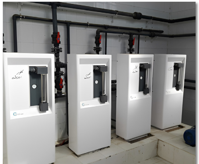
Sharki Water Treatment Station
