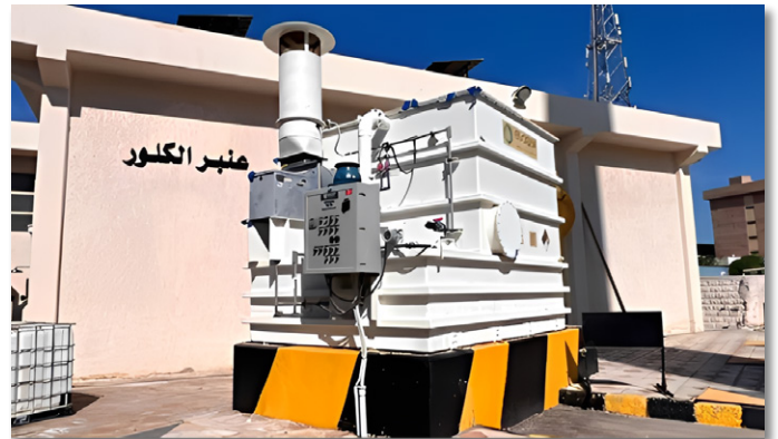
Sharki Water Treatment Station
