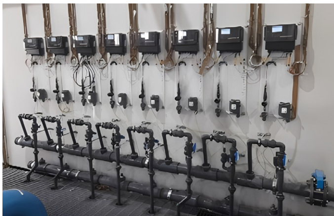
Gas Chlorination at Bahr El Bakar Project
