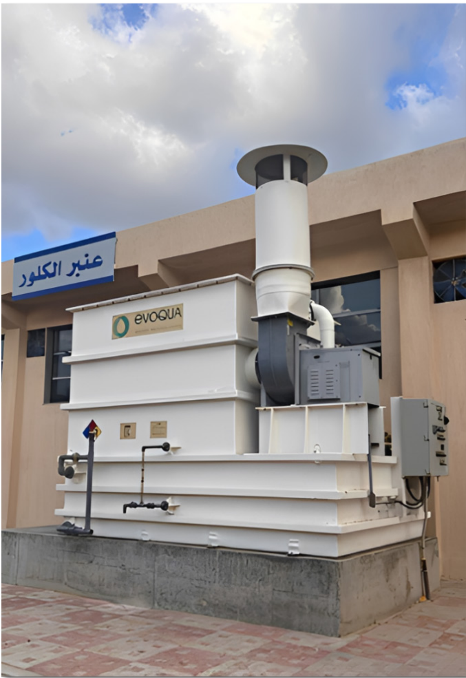
Seyouf Water Treatment Station
