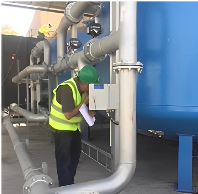
Filtration System at Iraq
