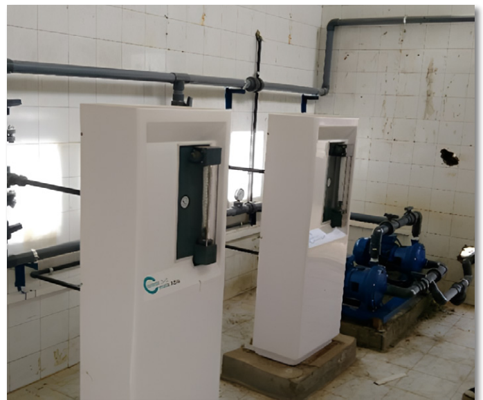
Hawamdeya Water Treatment Station
