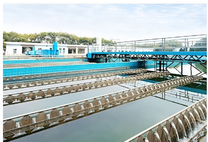
MBBR Sewage Treatment Plant
