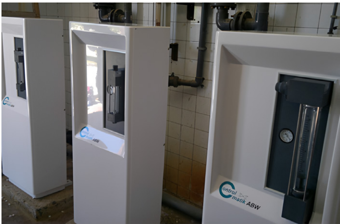
East Antara Water Treatment Station
