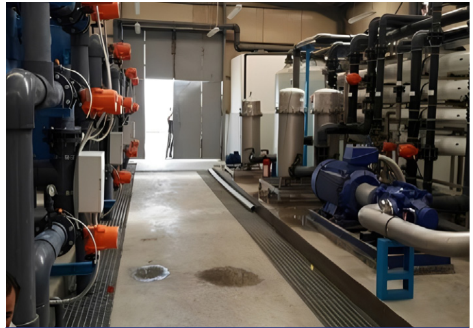
High Brackish Reverse Osmosis
