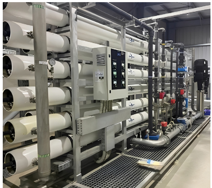
Brackish Reverse Osmosis
