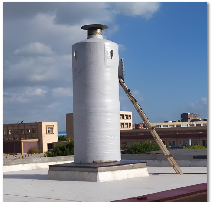
Mansheya Water Treatment Station
