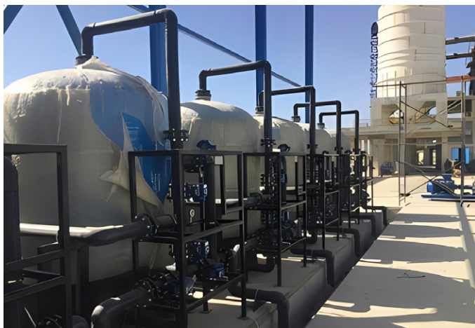
Pre-treatment Filtration System for Foreign Company
