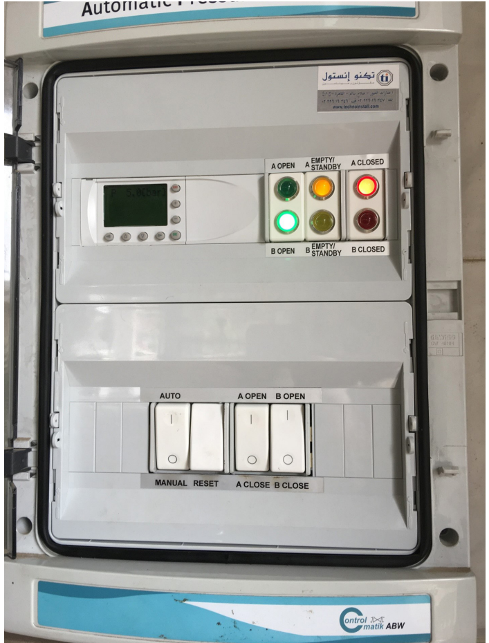
Ismailia Water Treatment Station
