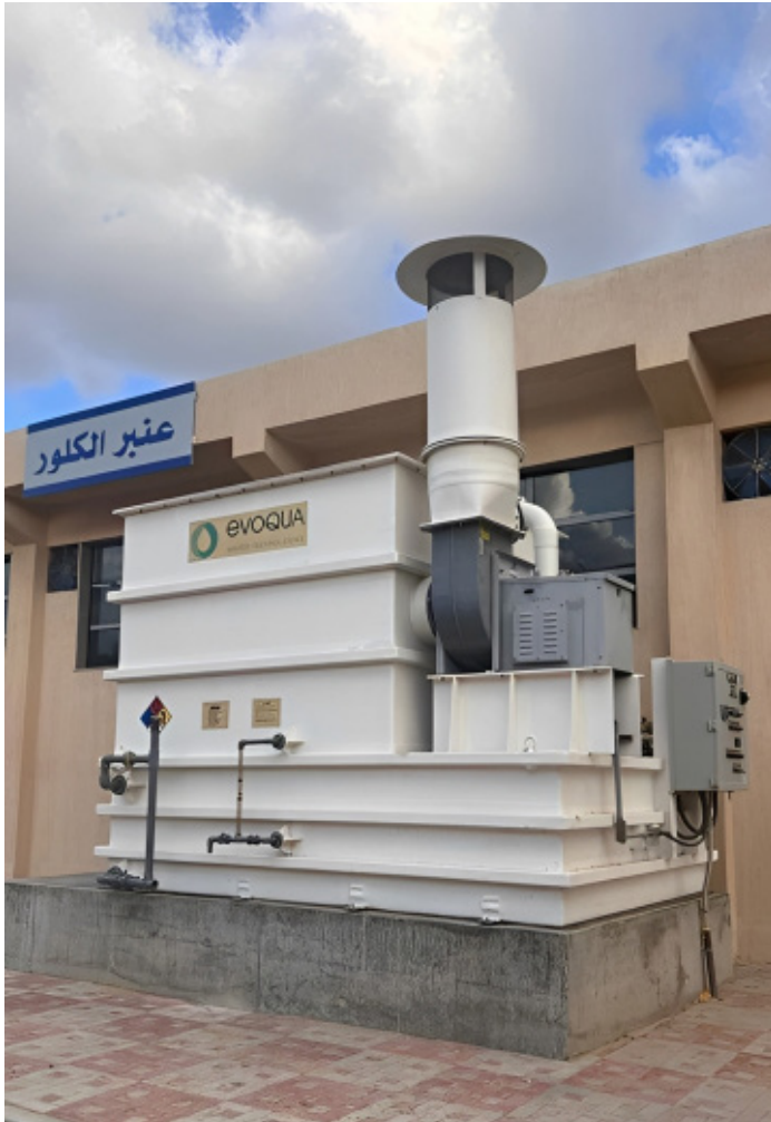
Seyouf Water Treatment Station
