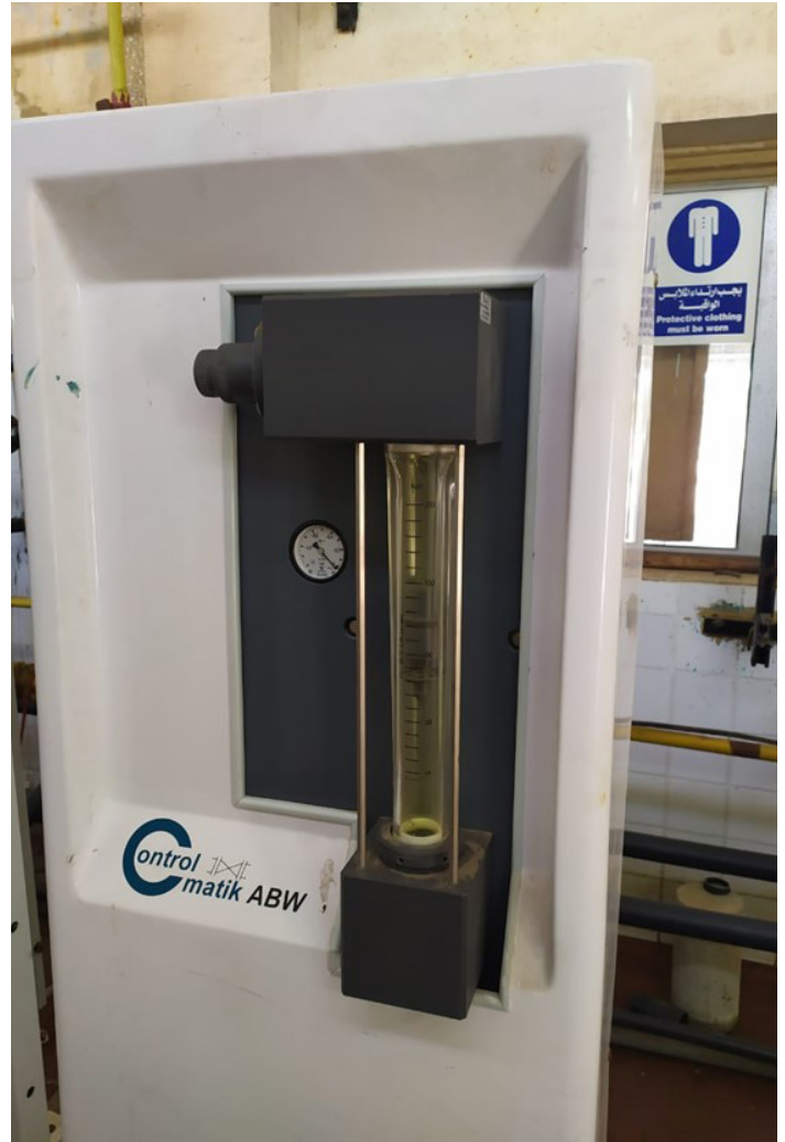
Supply & Installation of 4 complete chlorine gas injection systems 200 kg/hr. in Embaba WTS for Giza WTC.
