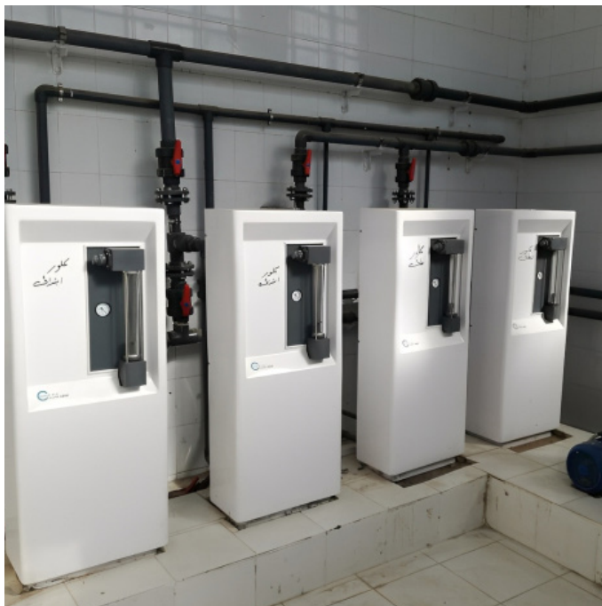
Dar Al Salam Water Treatment Station
