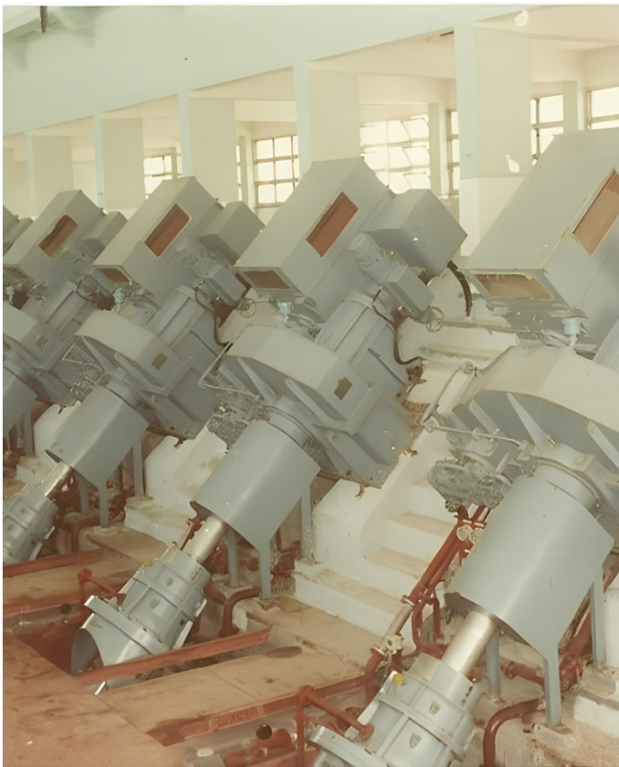
EL SALAM CANAL PUMPING STATIONS 1, 2 & 3 - TRANSFORMER STATIONS 1, 2
