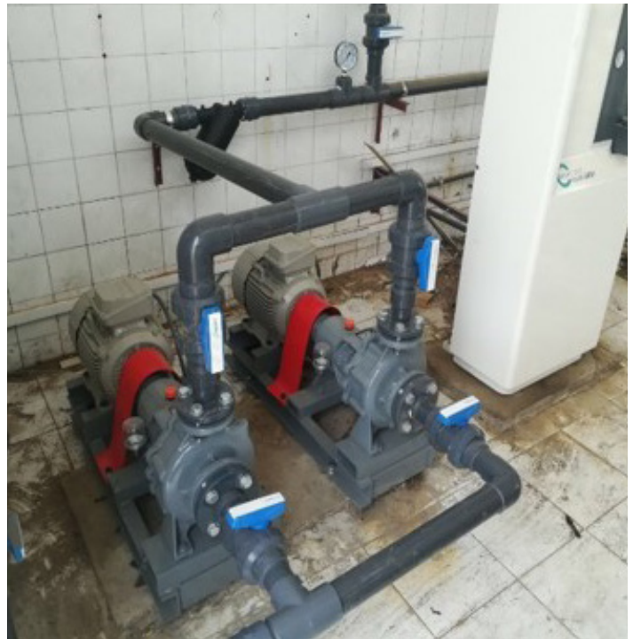
Badrashen Water Treatment Station
