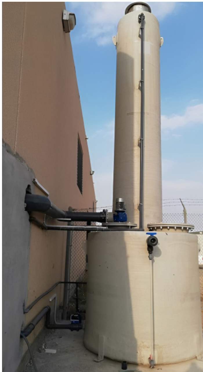
Baten Water treatment Station – KSA
