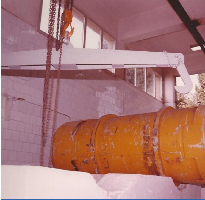
KOHAFA WATER TREATMENT PLANT
