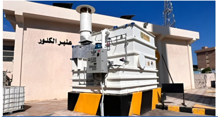
Sharki Water Treatment Station
