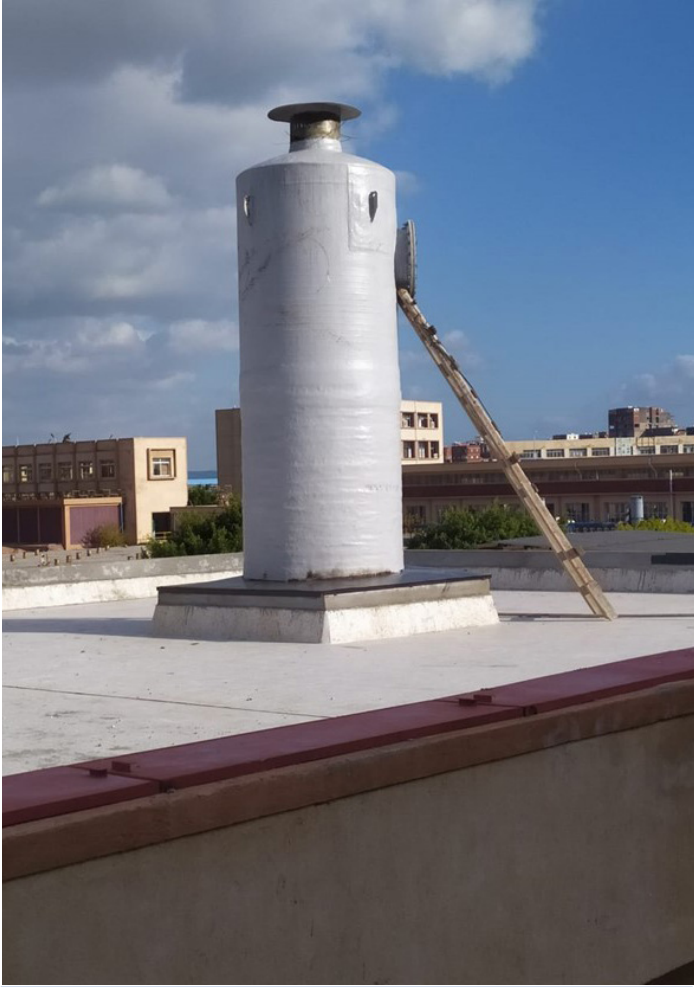
Mansheya Water treatment station
