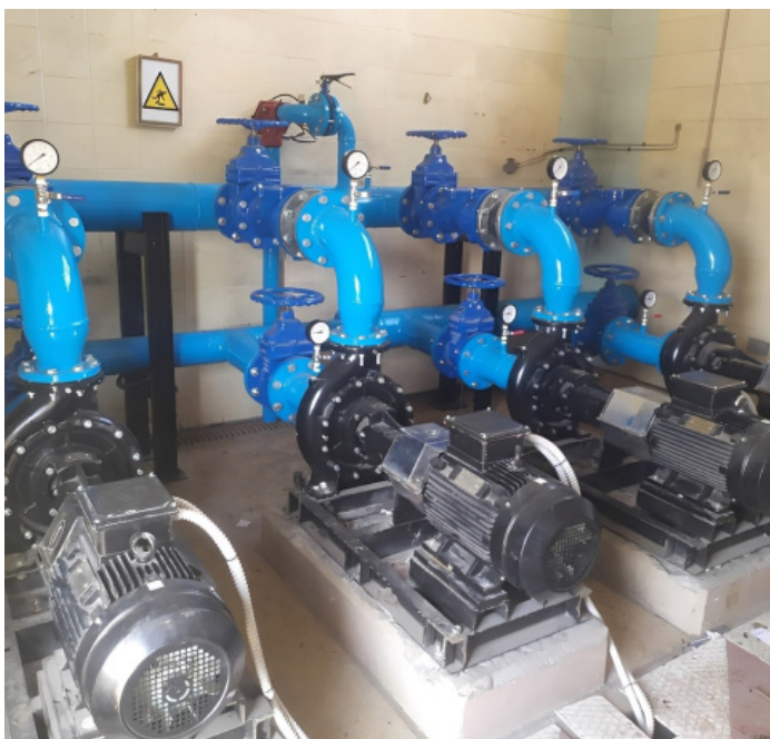
Mansheya Water Treatment Station
