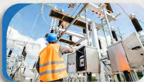
UGL Power Up To 400 kV
