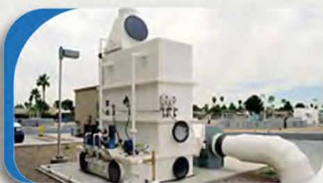
Water Treatment Systems
