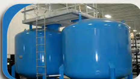
Ion Exchange Systems
