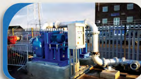
Eleven Pumping Station
