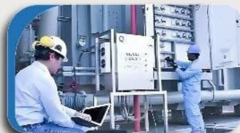
Transformer Testing Services
