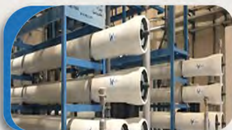
Reverse Osmosis Plants
