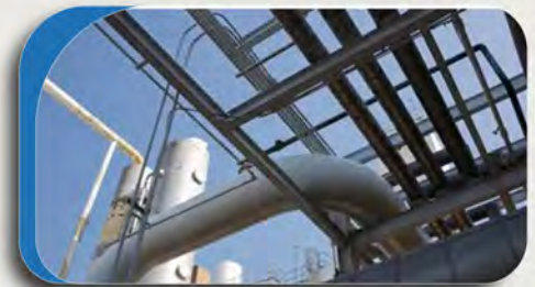
Wastewater Treatment Systems
