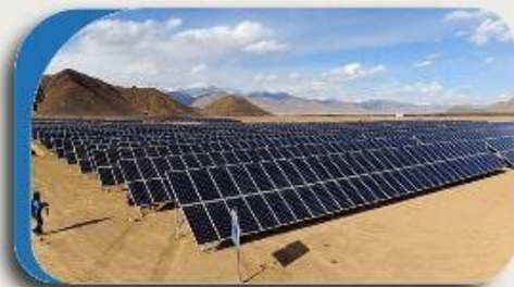
Solar Power System
