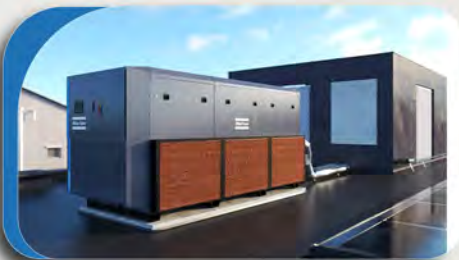
Water Cooled Chiller
