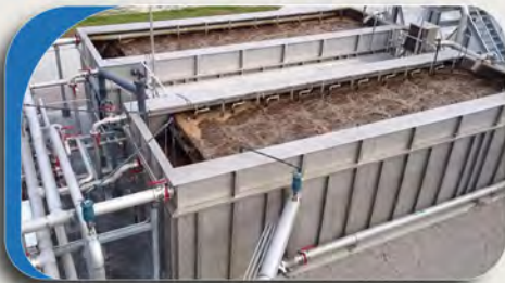
Membrane Bioreactor (MBR)
