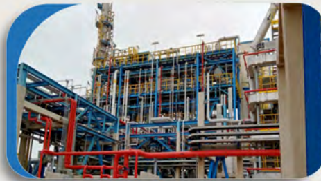
Stainless Steel Pipes
