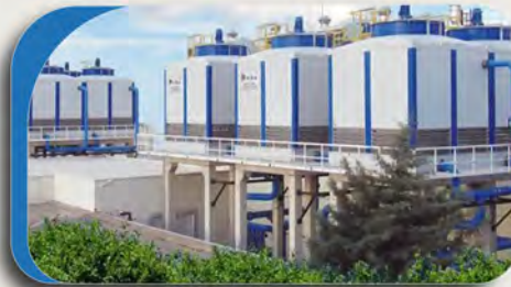
Water Cooled Chiller
