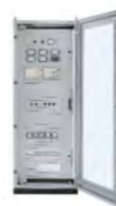
Control and Regulating Systems
