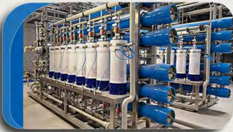
Ion Exchange Systems
