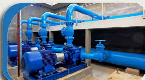
Water Supply and Treatment
