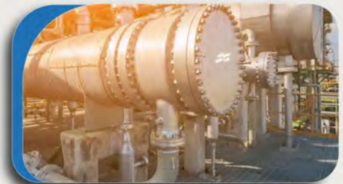
Water Cooled Chiller
