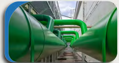
Water Cooled Chiller
