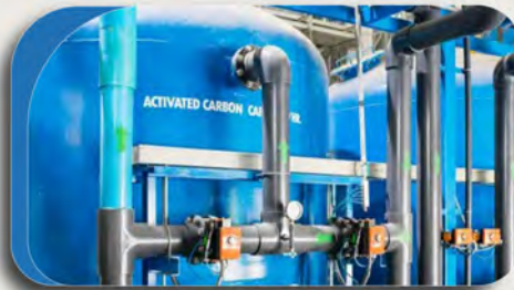
Wastewater Treatment Systems
