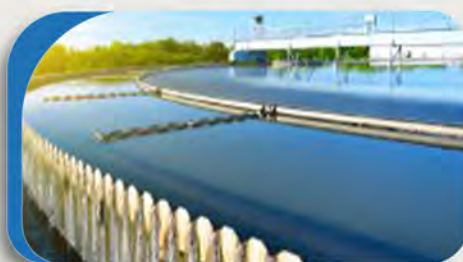
Water Treatment Systems
