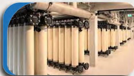
MuttENZ Water Treatment Plant
