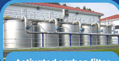
Activated carbon filter
