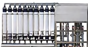
Ultrafiltration Water System
