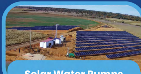
Solar Water Pumps
