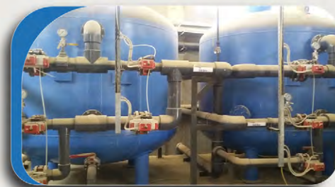
Water Desalination Plant
