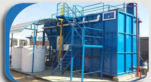
MBBR Treatment Compact Unit
