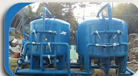
Iron Removal Filter Plants
