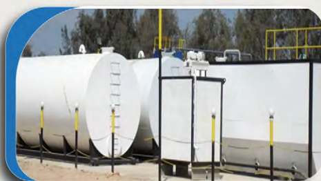
Wastewater Treatment Systems
