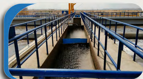
New Beni Suef City Sewage Treatment Plant – Egypt
