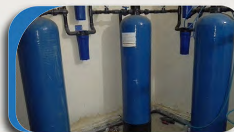
Water Desalination Plant – Hurgada
