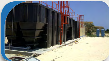
Wastewater Treatment Systems
