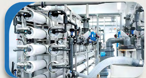
Design, Install, Commission of Projects
