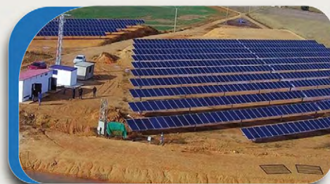
Solar Water Pumps
