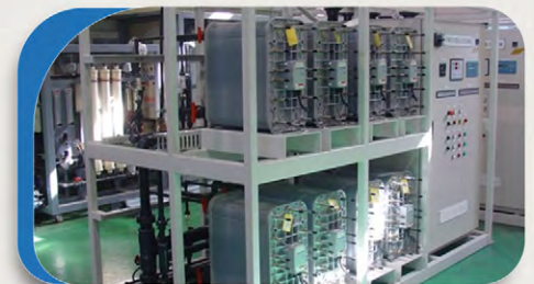
Ultrafiltration Water System
