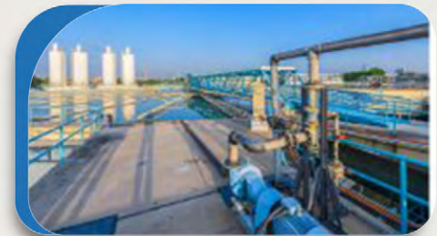
Water Treatment Stations
