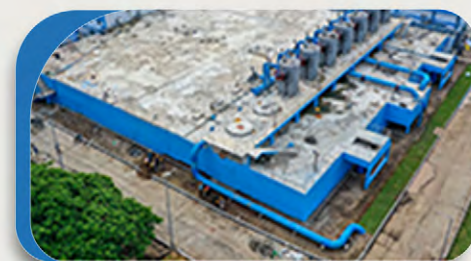
Koyambedu Water Reuse Plant
