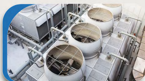
Refrigeration and Air Conditioning Systems
