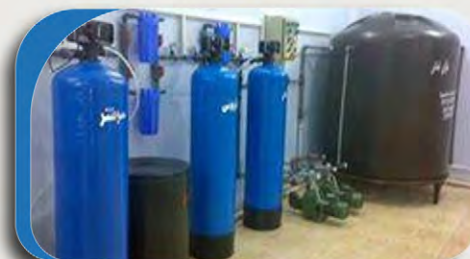
Reverse Osmosis Systems (RO)
