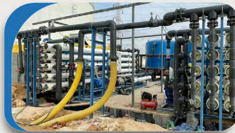
Reverse Osmosis Systems (RO)
