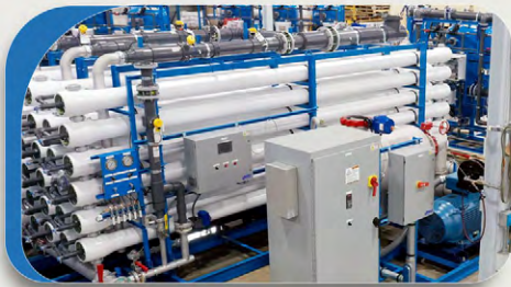
Reverse Osmosis Systems (RO)
