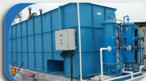
Membrane Bioreactor (MBR)
