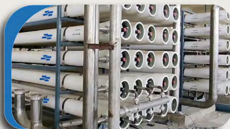
Reverse Osmosis Systems (RO)
