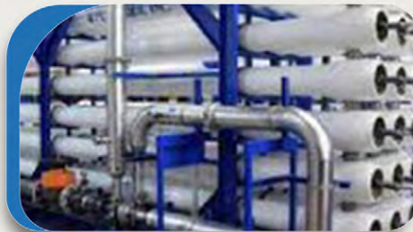
Industrial Wastewater Treatment Plants
