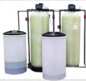
Softener Water Systems
